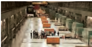
Robert-Bourassa generating station
